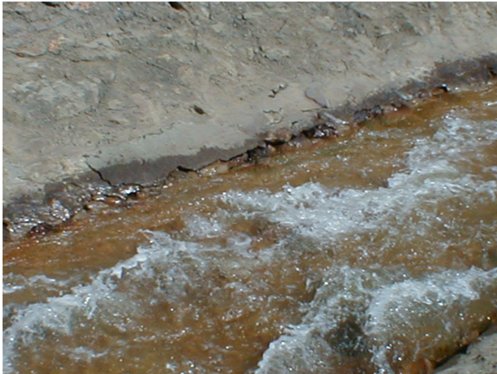
Figure 2: Typical surface condition, Willow Creek at Creede flume.
